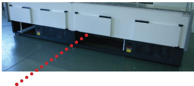
location of the condenser
